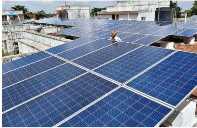
The scheme has facilitated the installation of 4,946 MW of rooftop solar capacity till July 2025 across States and Union Territories.
